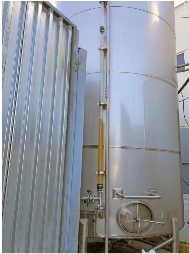
Image 3. The sight glass on this trub waste storage tank helps manage filling and emptying needs.
