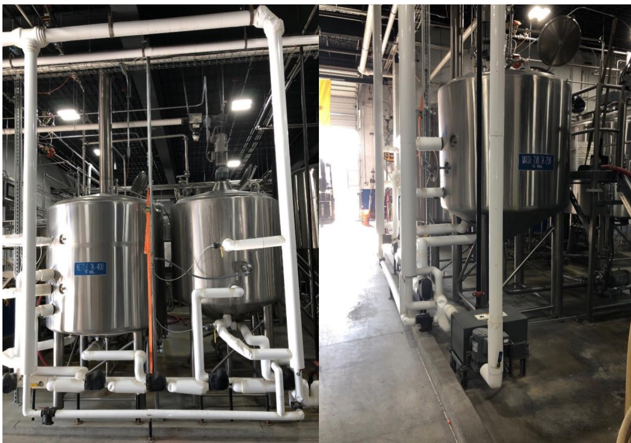
Figure 1. Left: Steam supply line at top of image with condensate system and steam traps depicted in the lower right-hand side; Figure 2. Right: an example of a condensate return system.
